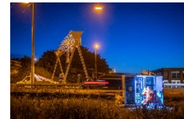
Intelligent Road Side Units
